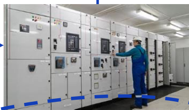
Distribution and control Board
